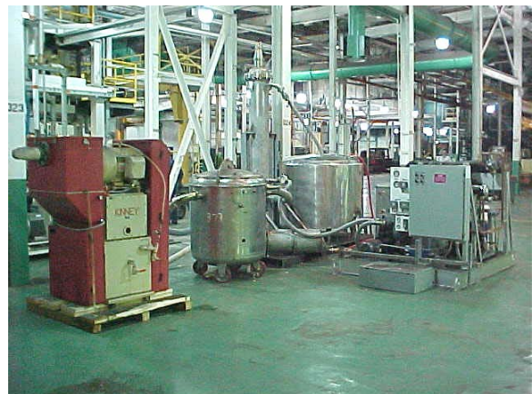
Figure 2-8 Hormel Vacuum Assist System
