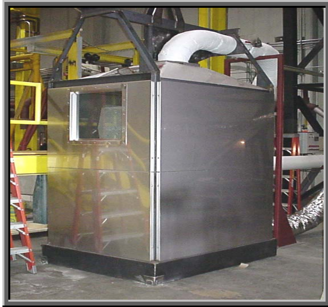
Figure 2a Technikon Research Foundry Emission Collection Hood
