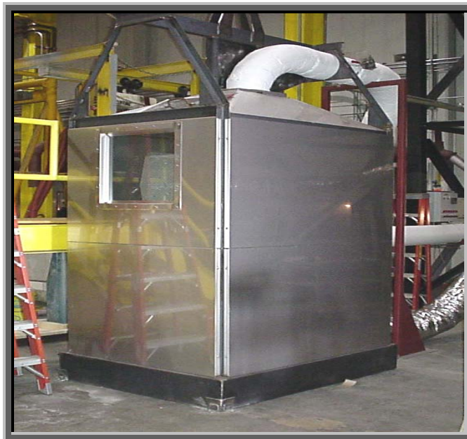
Figure 2a Technikon Research Foundry Emission Collection Hood
