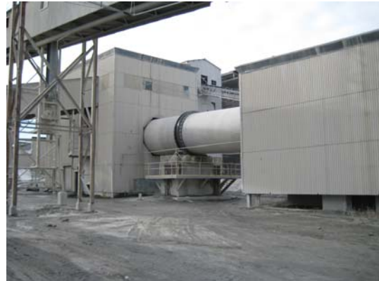
Figure 3. Machine that dries crushed and screened core sand.
