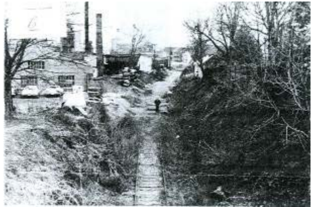
Photo 4: A view looking east from atop the old bridge in Photo 2. Note that this photo is a "before" and Photo 1 is an "after" taken from approximately the same location.
