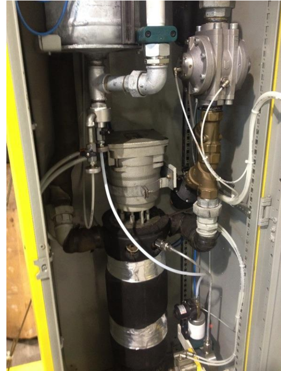
Internal view showing vaporizer
