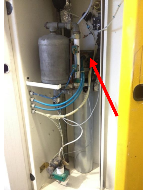
Internal view showing vaporizer
